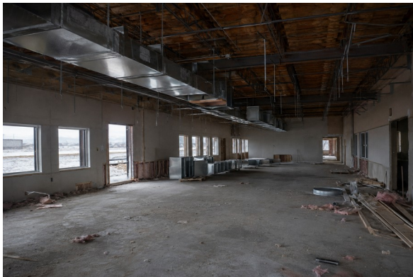
D03-02 - HVAC. Only the east main distribution run is installed; empty hangers continue west. COR field estimate: 30% installed versus 60% claimed. COR mark: /s/ Jack Raiden, 26 Aug 2027.
