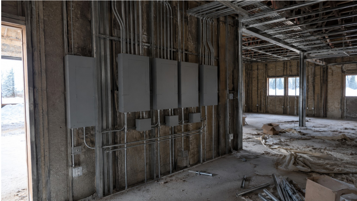
D03-01 - Electrical. Panels, feeders and branch-conduit work installed in Gallery E-14. COR field estimate: 52% installed versus 65% claimed. COR mark: /s/ Jack Raiden, 26 Aug 2027.
