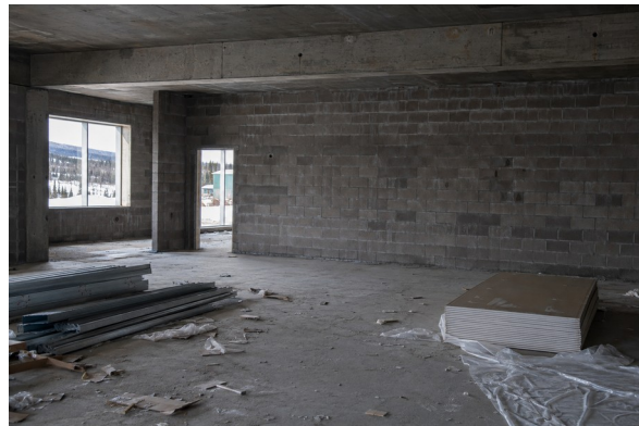
D03-03 - Drywall. Scheduled corridor remains bare with no metal framing or gypsum-board installation. COR field estimate: 0% installed versus 25% claimed. COR mark: /s/ Jack Raiden, 26 Aug 2027.
